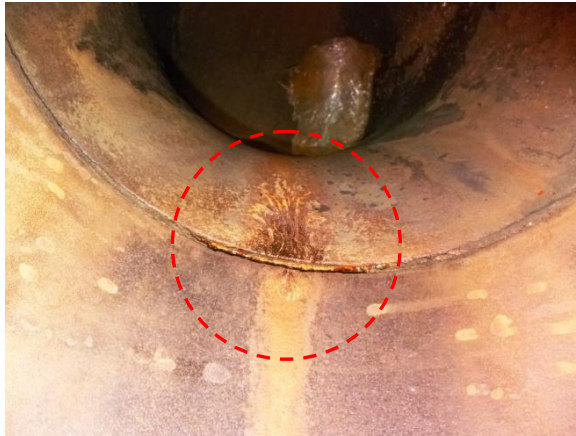
Lower part of the pipework (six o' clock position- Localised Root Defect)
