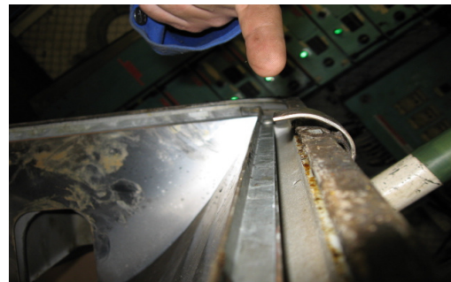
CLIP MECHANISM (INADEQUATE)
