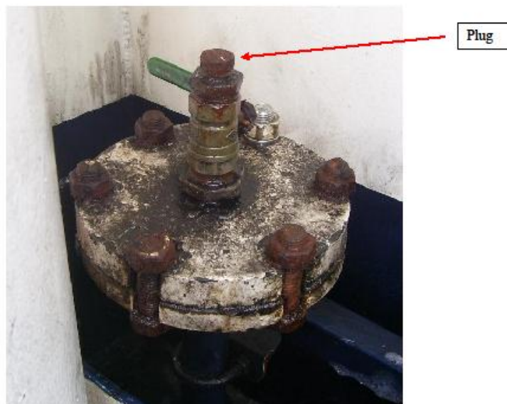
Starboard Waste Oil Connection
