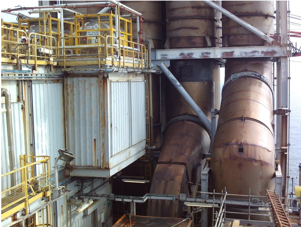
Position of helifuel tanks and exhaust ducting
