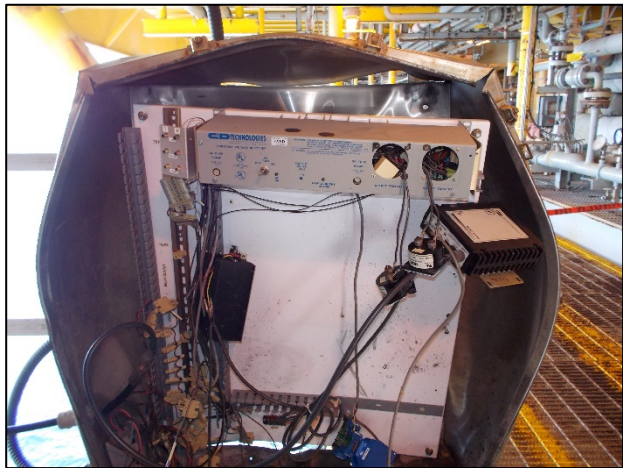
Remote Terminal Unit Panel
