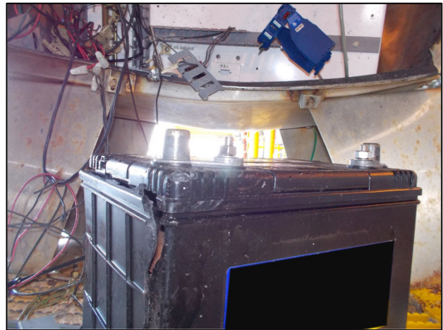
Overcharged 12 Volt Battery
