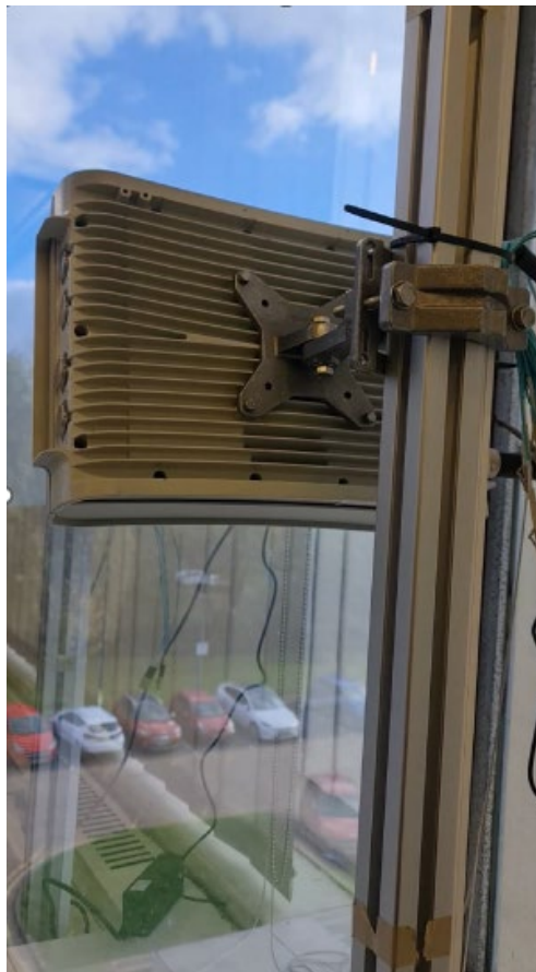
Figure 6-1: RunEL RU installed in the lab pointing outside the Brunel University
