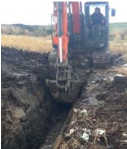
The power of modern diggers allows us to get to the source of the water, which was not accessible to our forebearers.
