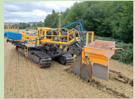
The scheme was installed with a drainage plough in good conditions. There was minimal surface disturbance
