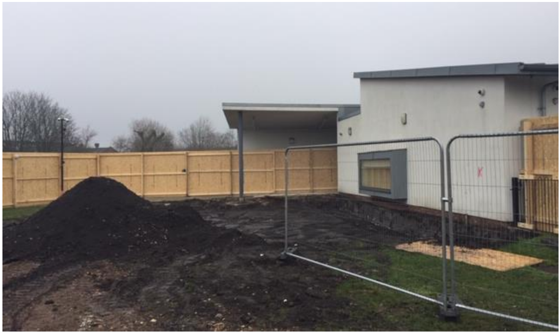
Further reduced level dig for excavations to new extension classroom including spoil heap from removal
