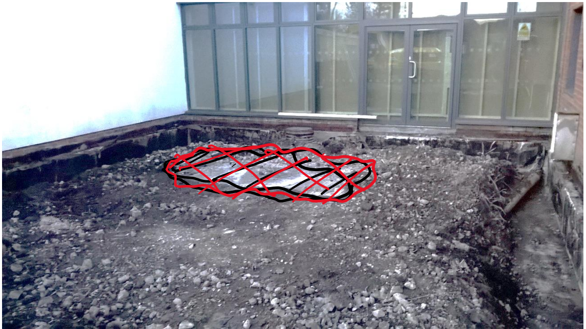
Unforeseen reinforced concrete slab discovered below courtyard paving during excavations
