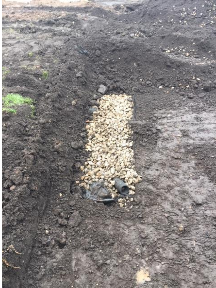
Existing land drains discovered in area of new extension
