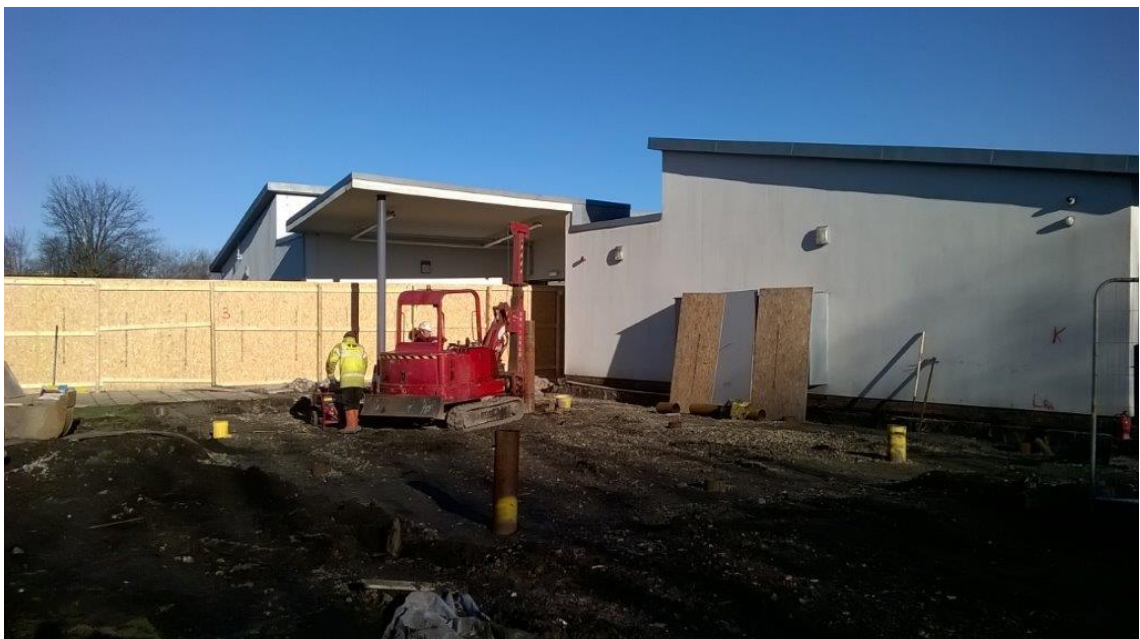
Piling Rig to extension classroom area (installed piles visible by yellow markings)
