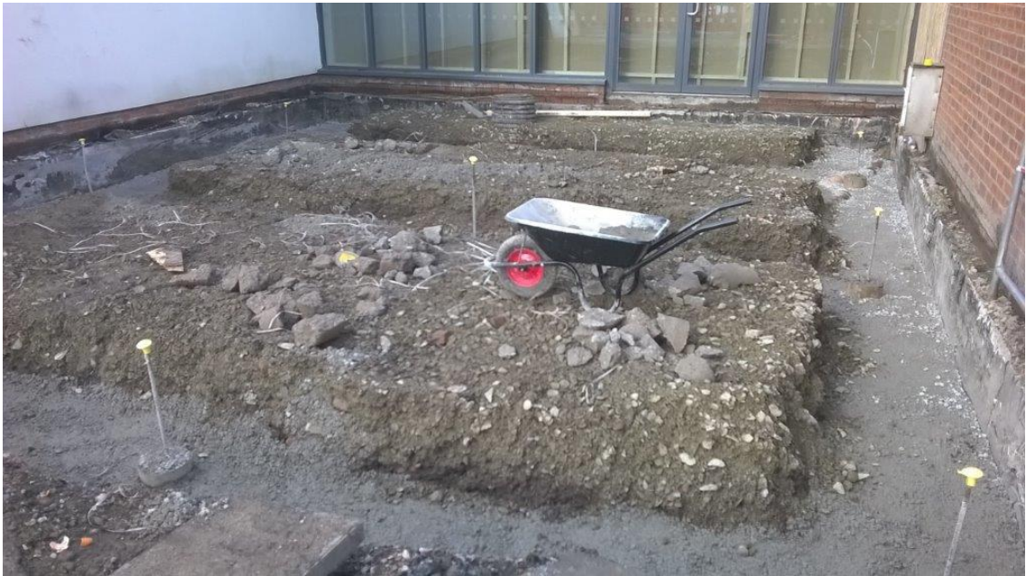
Reduced level dig to infill classroom and blinding to new ground beams. Pile heads just visible.
