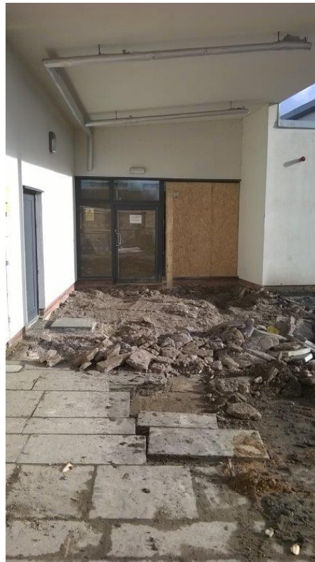
Closure of fire escape and protection to Assistant Head teacher's office windows. (Internal hoarding installed to doorway – not visible in photo)
