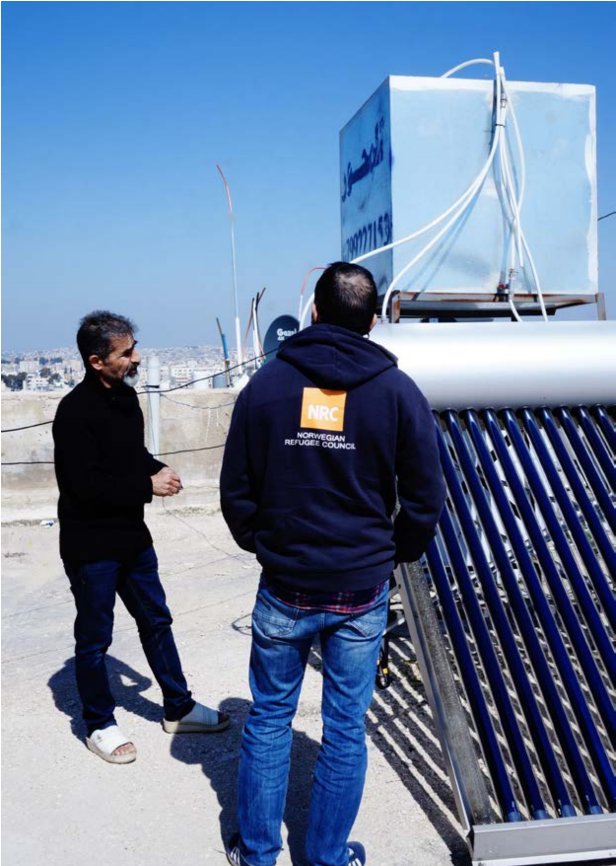
Reducing Poverty through Renewable Energy for Refugees (RE4R) Project, Solar Water Heater installation. © Shatha AbuOdeh/NRC
