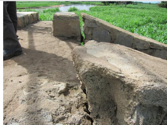
L. Foot Bridge Crack
