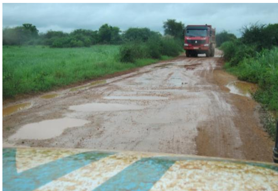
A. Metar Road (in Bad condition)
