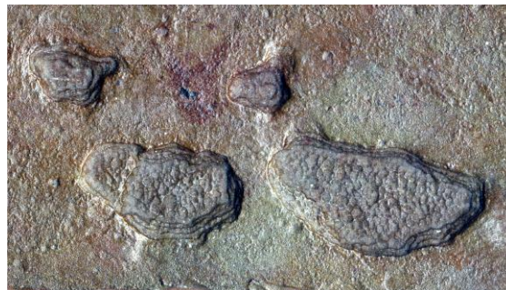
Pitting Corrosion caused by SRB
