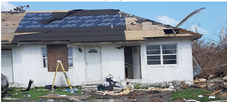
Example of a house with roofing damage in Murphey Town. Work is underway to make repairs. Note that damage is variable.
