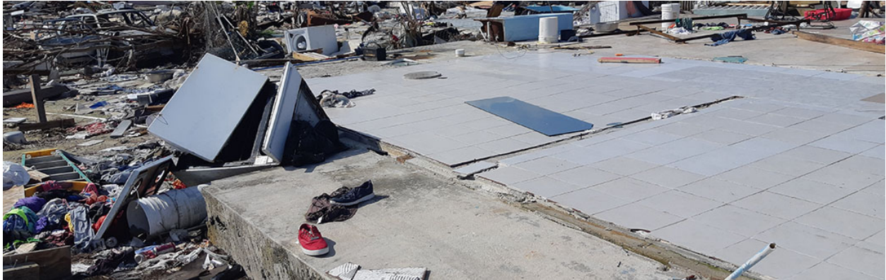
Example of the slab remaining from a destroyed shelter in Mudd. Remains of multiple rooms can be seen.
