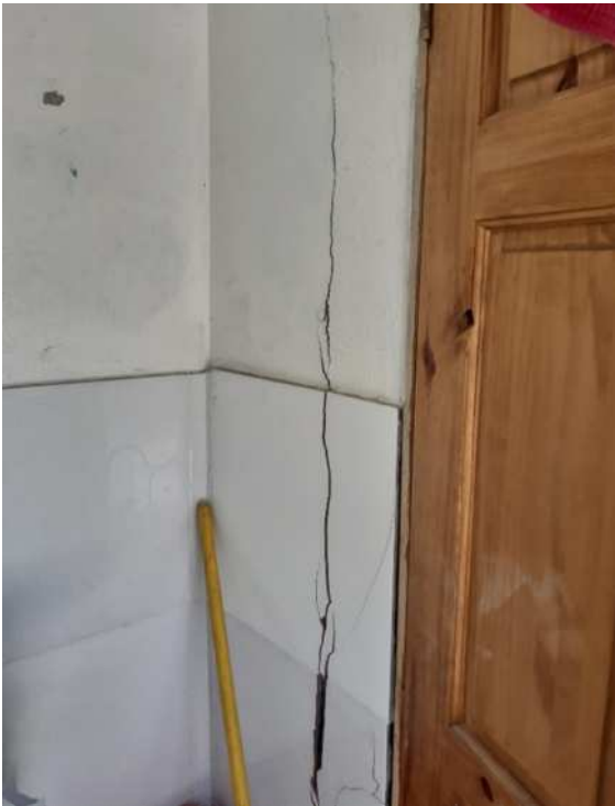
Figure 12 - Cracked and leaning wall in Building 5
