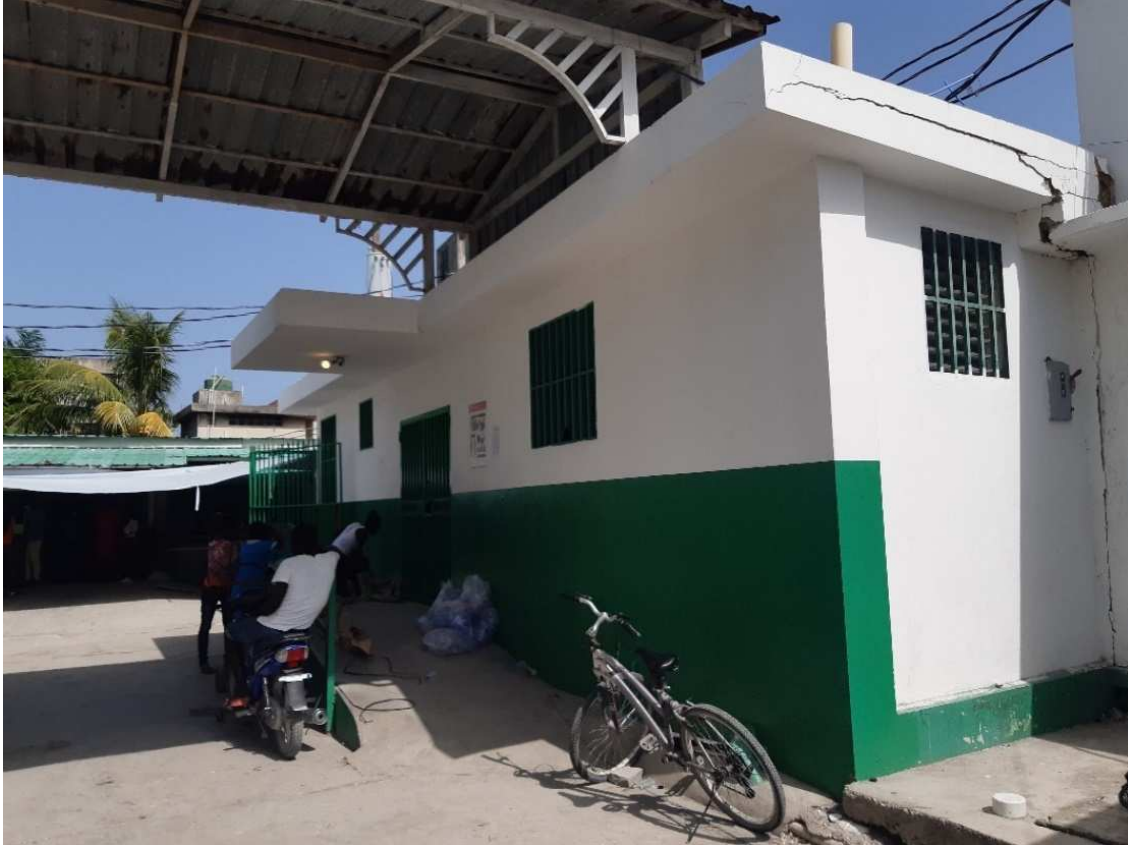
Figure 15 - Building 6, image shows cracking to the external edge of the roof slab
