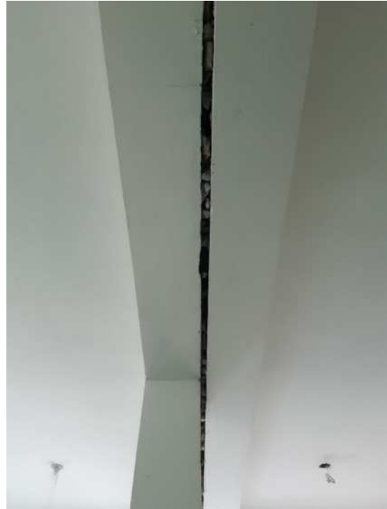
Figure 30 - Cracking along the movement joint in building 15
