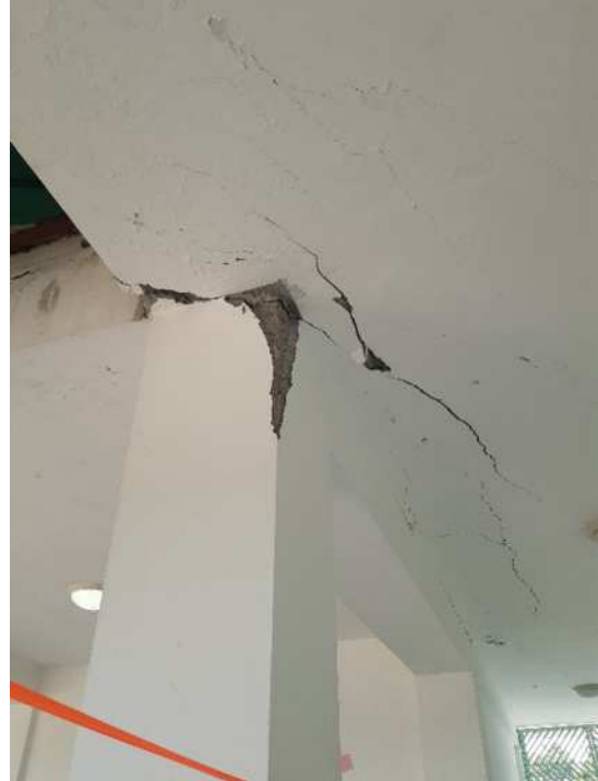
Figure 70 - Cracking around the column head and slab
