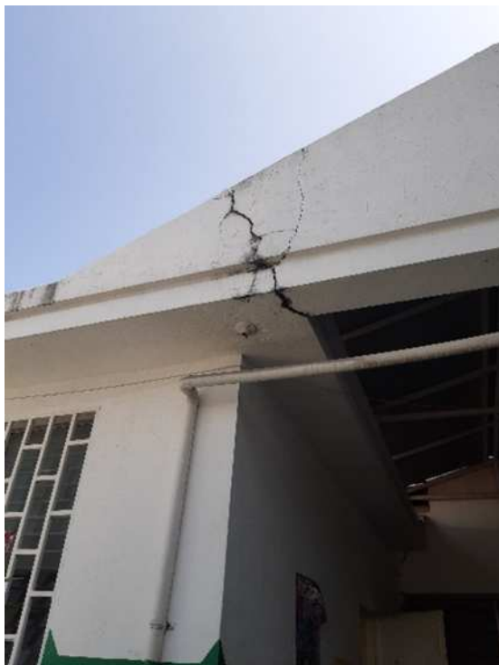
Figure 22 - Crack in the entrance arch
