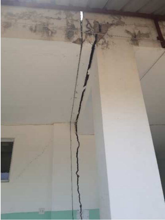
Figure 69 - Movement joint cracking resulting in loose fill
