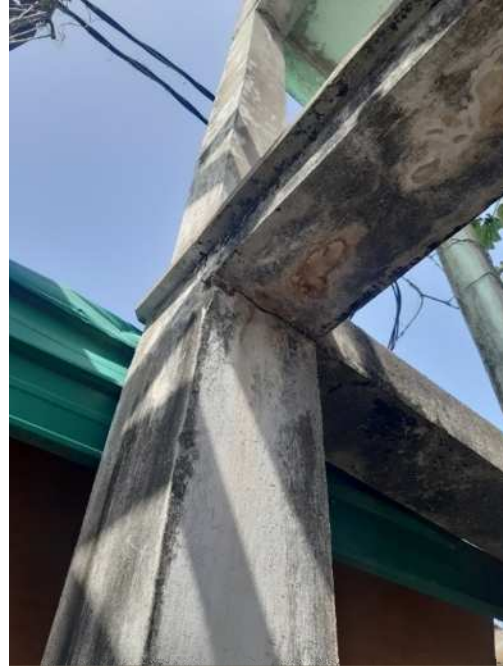
Figure 9 - Cracking between the beam and column joints
