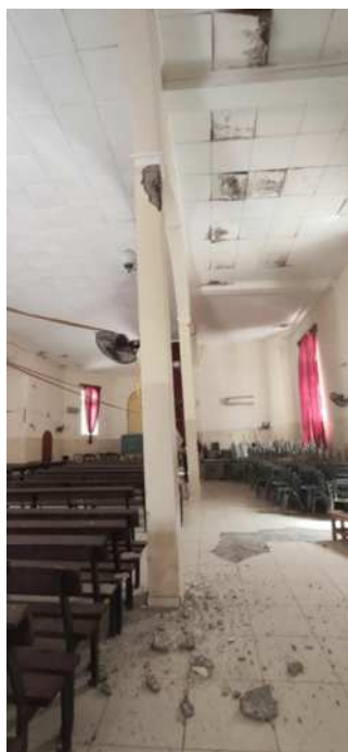
Figure 39 - Extensive structural cracking observed from inside the “auditorium” building
