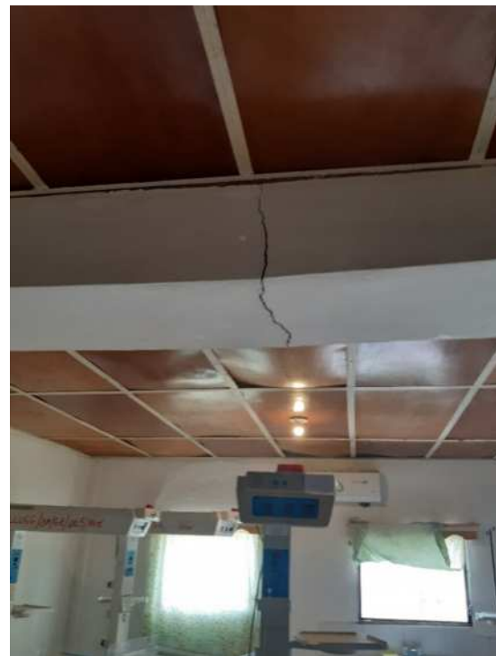
Figure 23 - Crack in a supporting beam
