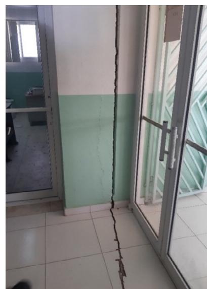
Figure 68 - Movement joint cracking
