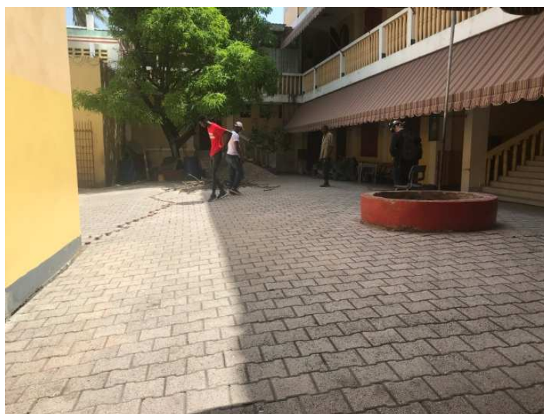
Figure 37 - Building 21 courtyard heave
