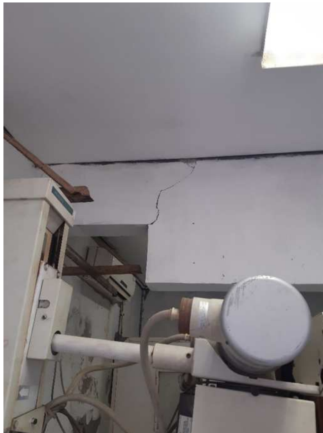
Figure 17 - Cracking of the supporting beam
