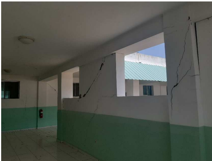
Figure 71 - Column cracking and short column shear crack
