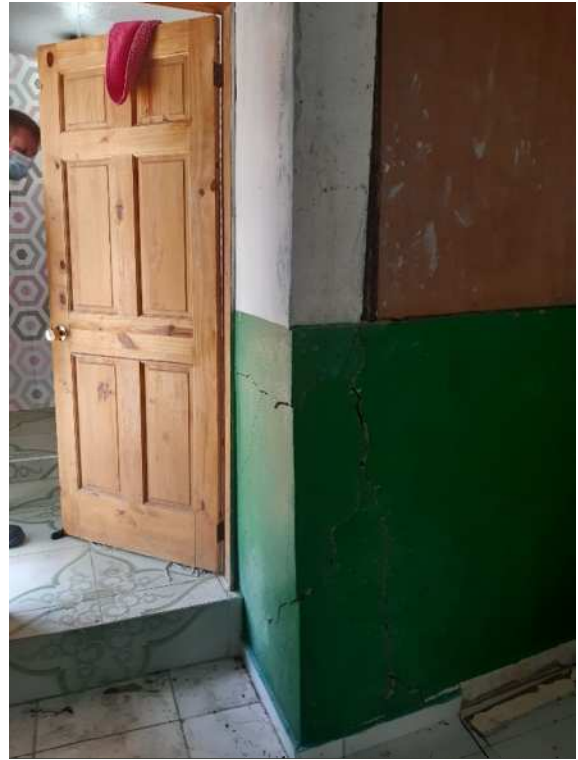
Figure 13 - Cracked and leaning wall in Building 5
