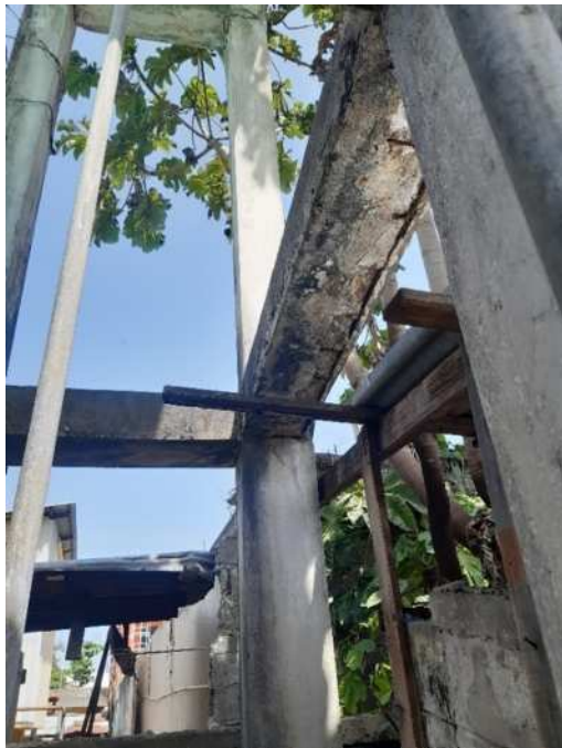
Figure 10 - Spalling of the concrete on the beam
