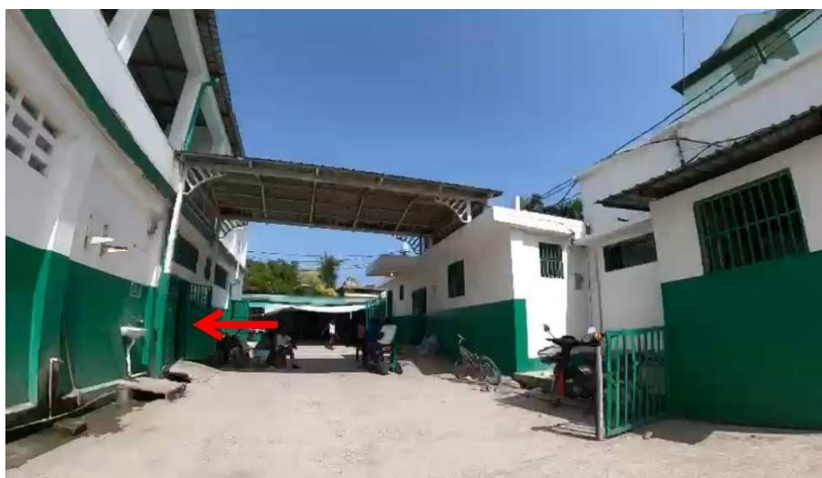
Figure 6 - Access into the room with a damaged column is indicated by the red arrow.
