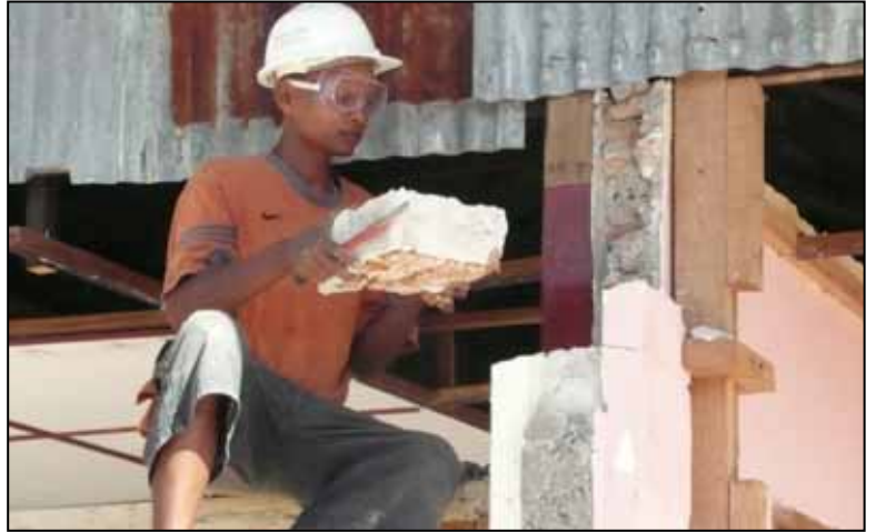
Masonry columns realized with poor quality bricks and without any connection to the wall.
