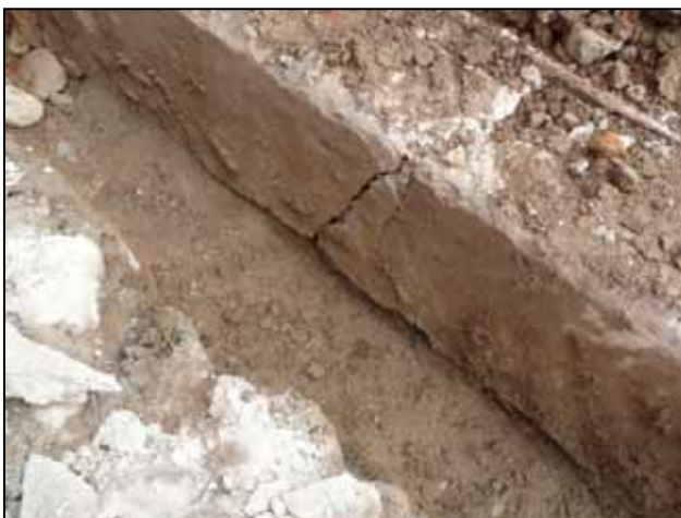
Very poor quality foundations
