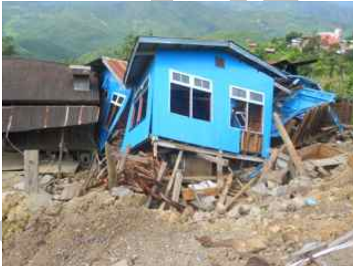
Landslide damaged house Chin State. Photo courtesy of IOM
