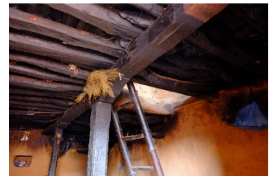
Burnt wood structure: this process protects the surface of the wood and slows the spread of fire, Dolakha, 2015 – ©CRAterre
