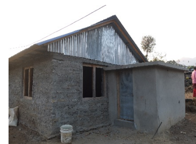
Addition of an extra room, in direct contact with the « core » house. The risk is high of damages, in case of earthquake – ©HRRP
