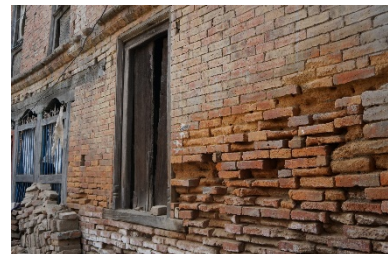
Erosion of bais of burnt bricks due to capillarity/ lack of proper drainage, Bakhtapur, 2016 ©CRAterre
