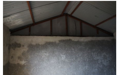
Finished house covered with CGI sheets on a metal structure, without ventilation, wall covered with cement plaster: indoor air condenses in the walls and roof. Cool materials radiate. Dhapa, 2019—©CRAterre
