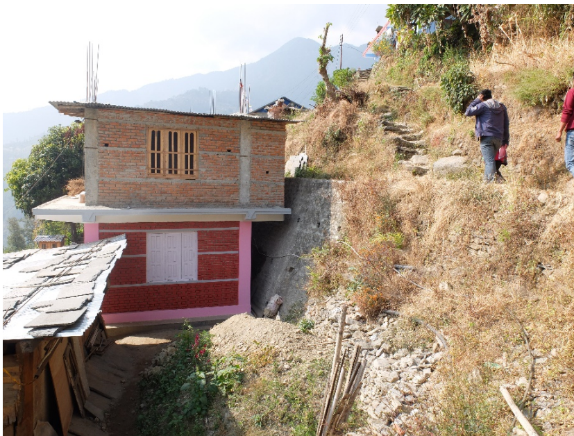
Hazardous vertical extension, asymmetrical load descent, exposed rebar on the roof (probably for future extension), Sindhupalchwok, 2018 – ©CRAterre
