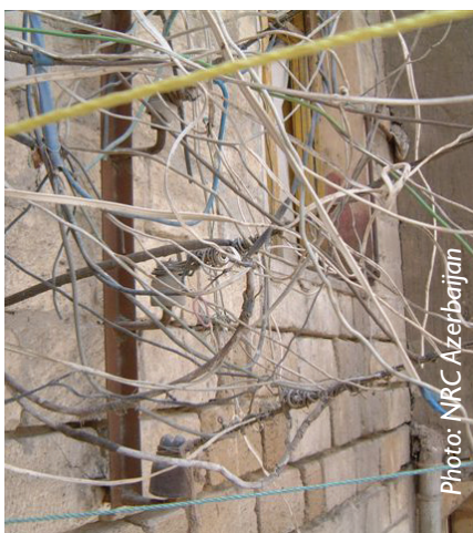
Wiring before upgrade
