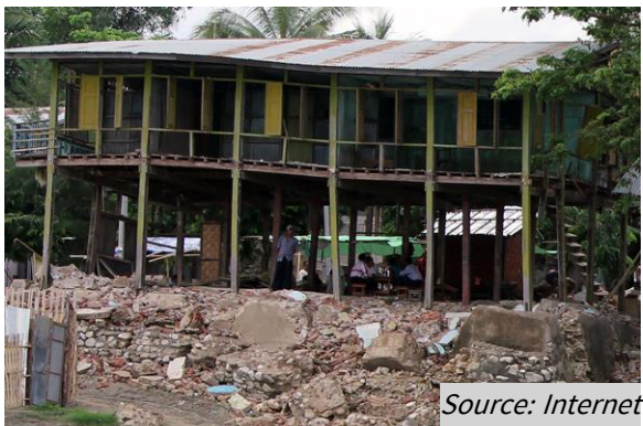
Figure 70: Failure of interior and/or exterior walls
