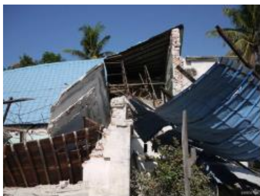
Figure 2: Housing Damages Due to Thabeikyin Earthquake
