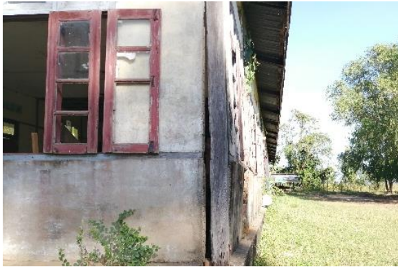
Figure 66: Slight separation of walls from timber post
