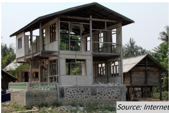
Figure 49: Failure of interior and exterior walls (Moderate)
