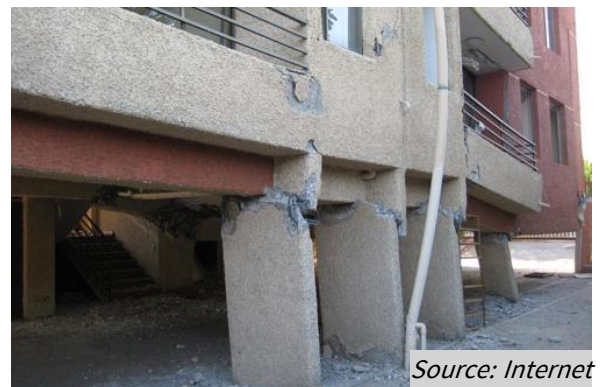
Figure 58: Subsidence of upper floors, and fracture of reinforcing bars(severe)
