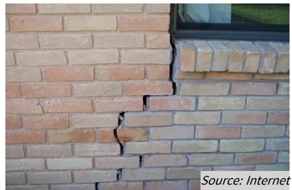
Figure 75: Cracks in bearing wall
