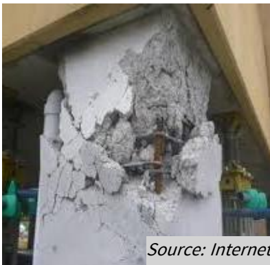
Figure 55: Reinforcing bars are exposed due to spalling of the covering concrete (Moderate)
