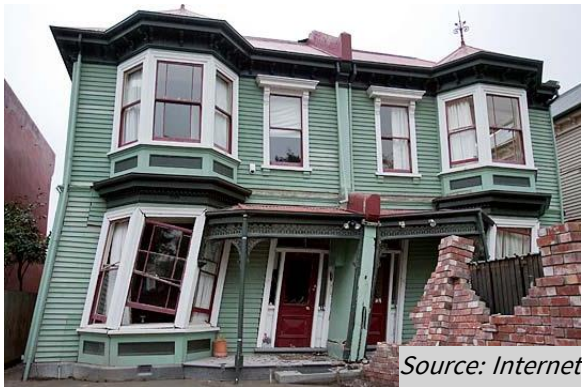
Figure 47: Inclination of building (Moderate)
