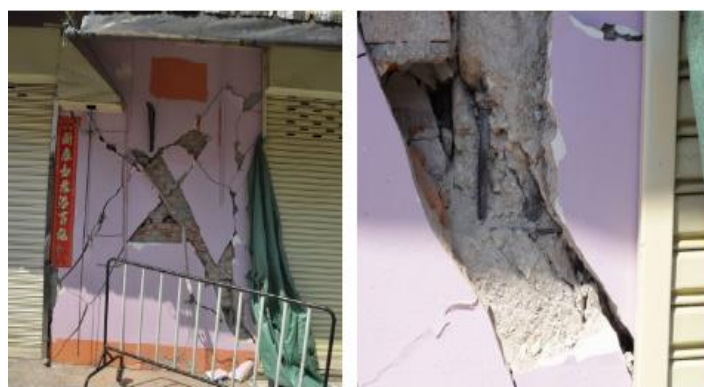
Figure 3: Housing Damages due to Tarlay Earthquake
