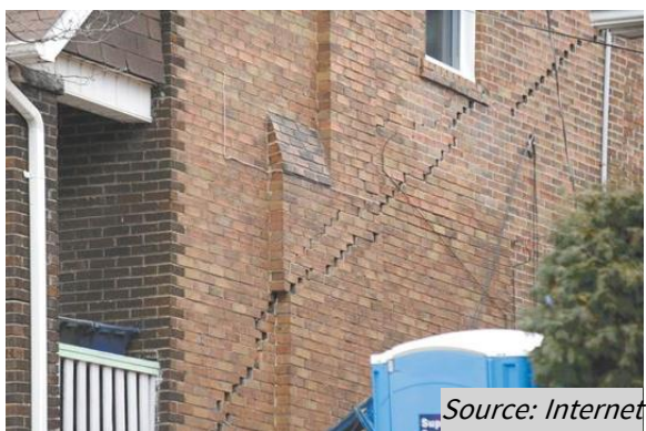
Figure 51: Wall crack in building (Moderate)
