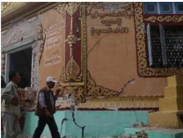
Figure 8: Post Earthquake Assessment after Tabeikyi Earthquake
