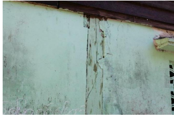
Figure 67: Minor cracks in structural elements
