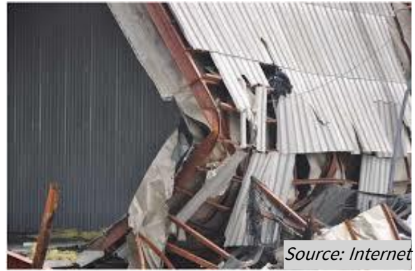
Figure 54: Damage in the vertical members (Severe)
