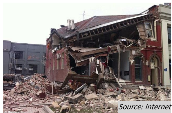
Figure 52: Partial Collapse (Severe)
