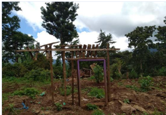
Figure 2 Example of damaged shelter in Eda Farfa (Kercha) by GOAL.
