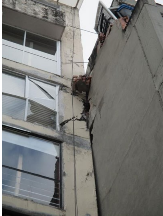
Figure 13: Example of damage caused by pounding buildings, Mexico City, October 2017
