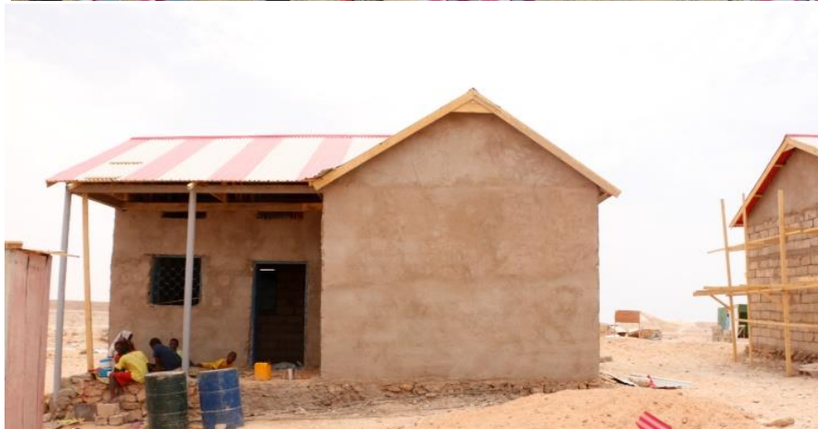
A shelter unit under construction in the relocation site in Girible settlement through owner driven approach.
