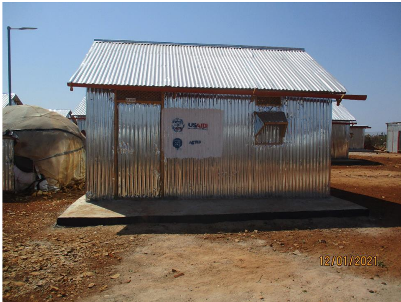
Photo: CGI transitional Shelter constructed by ACTED featuring a door, a window, and a cemented floor.
