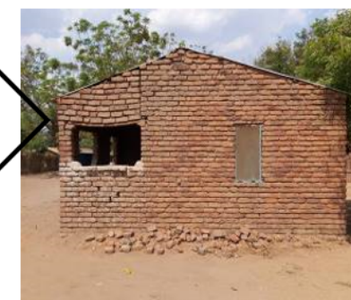
Side Gable CGI covered (burnt brick) Design – lintel failing due to heavy brick loading and lengthy span
