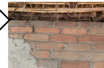
Missing wall plate for even distribution of load on the wall
