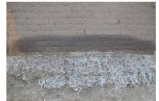
1. Absence of damp proof course. Moisture reduces wall resistance
