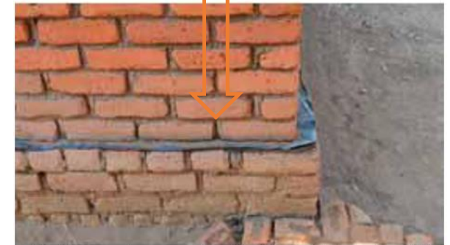
Plastic membrane protecting the wall from humidity in Masako, Dowa (bottom). © Jon Twingi
