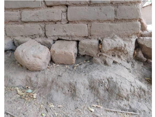
Wall starting on a header course on the ground without foundation
