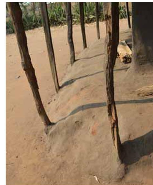
When wooden poles are in direct contact with the ground and are not regularly treated or replaced, they are vulnerable to rising damp and decomposition. Veranda in Lfidzi, Salima. © Jon Twingi
