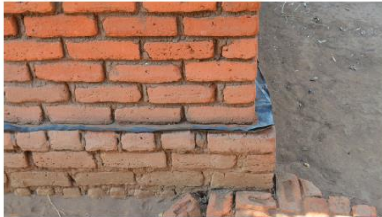
Plastic membrane protecting the wall from humidity in Masako, Dowa (bottom). © Jon Twingi
