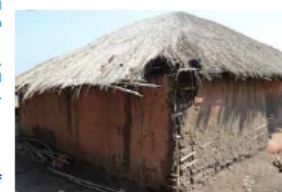
Maintenance of roofs is crucial to block water from penetrating the walls and to make them stay stable. House in Mwachenje, Karonga. © Jon Twigg
