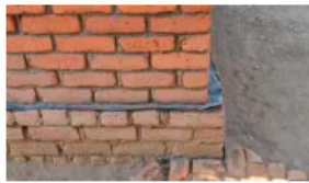
Plastic membrane protecting the wall from humidity in Mazako, Dowa (bottom). © Jon Twigg
