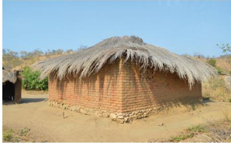
Stone foundation and plinth (Chimwendo, Karonga) protecting the walls from humidity and floods.
