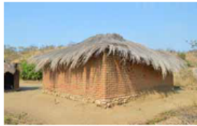
Stone foundation and plinth (Chimwendo, Karonga) protecting the walls from humidity and floods. © Jon Twigg
