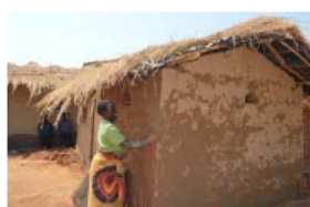
Women plastering her house with earth plaster in Nkhombe, Kasungu. © Jon Twingi.
