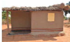
Thatched roofs are repaired when necessary. This house in Chome (Rumphi) presents thatch bundles which can be easily replaced when they get rotten. © Jon Twigg
