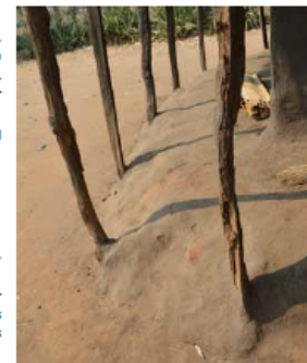
When wooden poles are in direct contact with the ground and are not regularly treated or replaced, they are vulnerable to rising damp and decomposition. Veranda in Lifizi, Salima. © Jon Twigg
