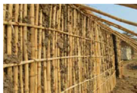
Wattle and daub house under construction in Chipite, Karonja. Bamboo framework and earth mortar. © Jon Twingi.
