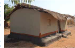
The earthen mounds are strengthened before the rainy season. The foundations are improved with an extra layer of mud. House in Chama, Dowa District. © Jon Twigg
