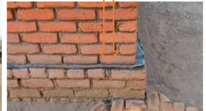
Plastic membrane protecting the wall from humidity in Masako, Dowa (bottom). © Jon Twingi
