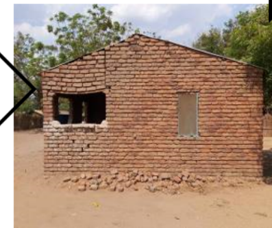
Side Gable CGI covered (burnt brick) Design – lintel failing due to heavy brick loading and lengthy span
