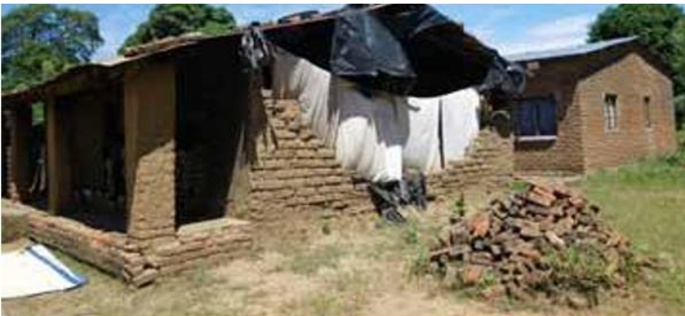
Unsupported masonry gables tend to fail in the out-of-plane direction in the event of an earthquake. This house's gable fell after the Karonga earthquake in 2009. © Sonia Molina
