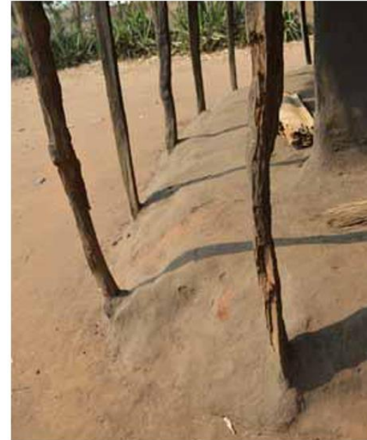
When wooden poles are in direct contact with the ground and are not regularly treated or replaced, they are vulnerable to rising damp and decomposition. Veranda in Lifidzi, Salima. © Jon Twingi
