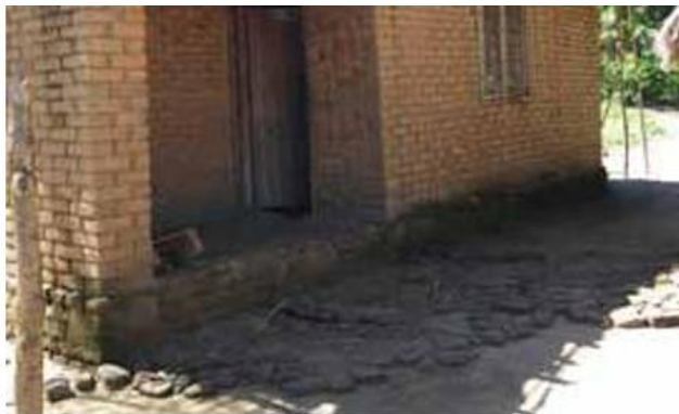
Raising dampness creates unhealthy living conditions inside the houses due to moisture. © Sonia Molina
