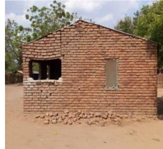
Side Gable CGI covered (burnt brick) Design – lintel failing due to heavy brick loading and lengthy span
