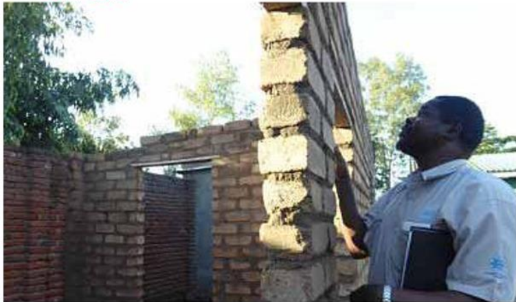
Walls with insufficient thickness and an important height are dangerous in the events of a disaster as they are not stable enough. CC - Ignasio Ngoma
