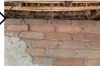
Missing wall plate for even distribution of load on the wall
