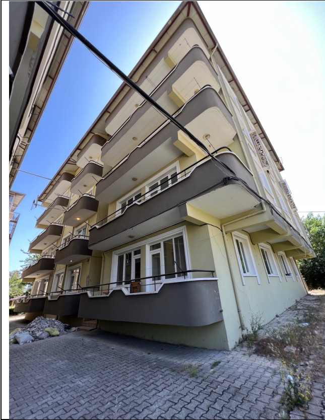
OUTSIDE On the building external walls are huge cracks to note on the plaster and cracks on columns. Some soil settlement is to note on the surrounding area of the building.
