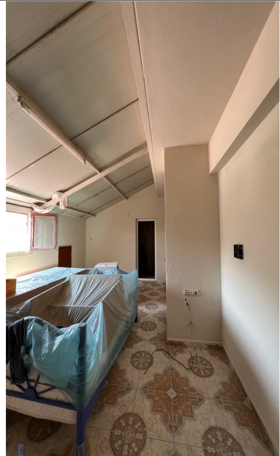
On an apartment below the roof, was no damage on the roof system observed
