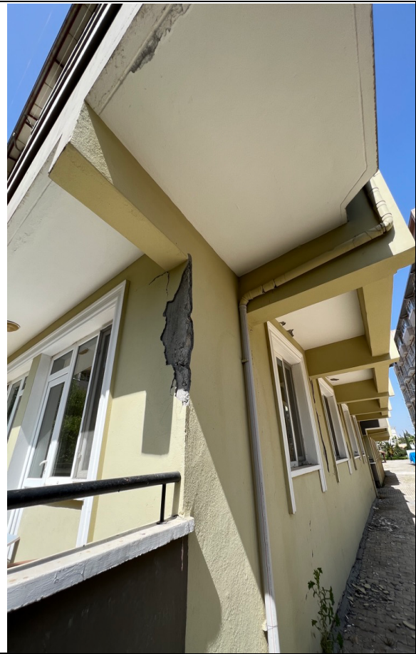
On the corner of the building was a crack on the column of the external wall observed
