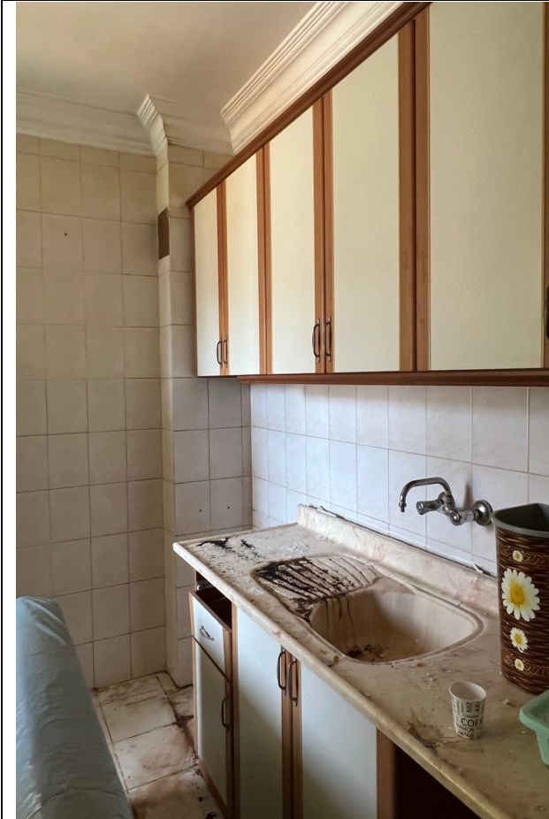
Inside the staff apartment were no structural damages observed, as the repair works are finished inside the apartments.
