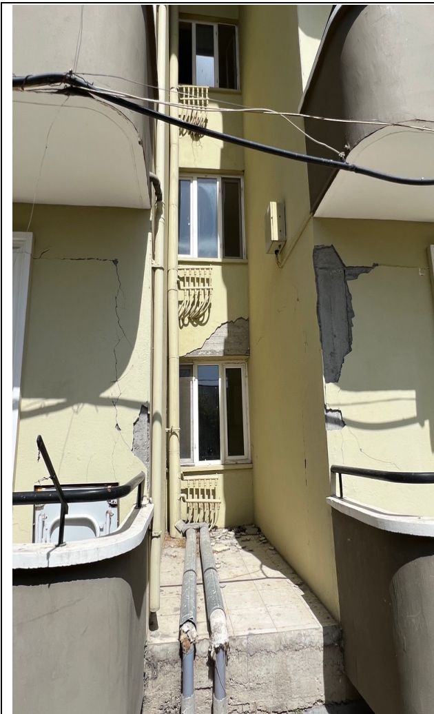
On another column of the external wall was also a crack observed (right side of the photo)
