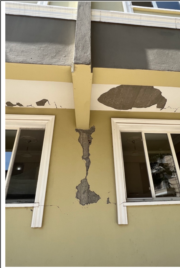
On another column of the external wall was also a crack observed
