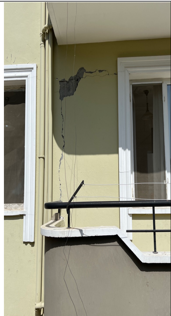
On another column of the external wall was also a crack observed
