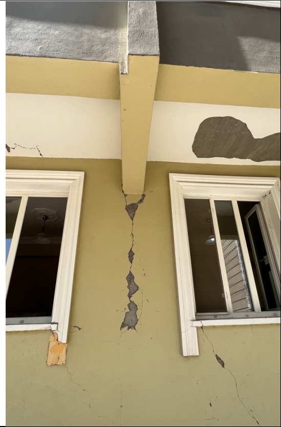
On a column of the external wall was a crack observed
