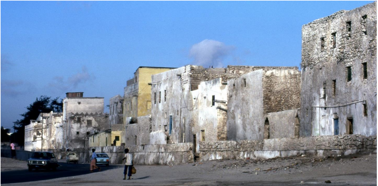
Use of coral stone in buildings of Mogadishu old town (CC - Franck Keillor)
