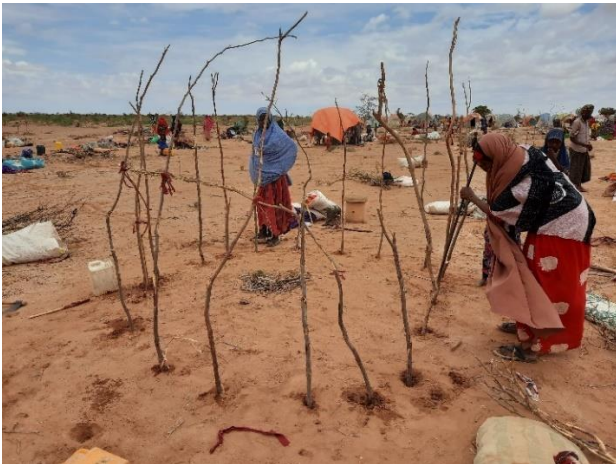
Construction of the structure of a buul with small section lumber (Doolow) (CC - Enrique Sevillano Gutiérrez - CRAterre)
