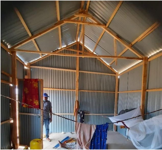
Use of imported sawn timber as framework in a shelter in Doolow, Jubaland (CC - Enrique Sevillano Gutiérrez - CRAterre)
