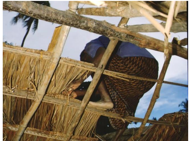
Use of lumber in the framework of a vegetal roof (Merca, Jubaland) (© Thierry Joffroy)
