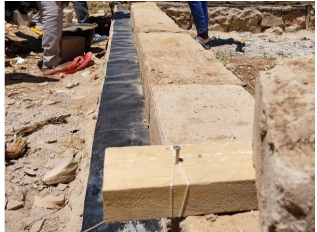
Anti-dump membrane between stone base and adobe elevation (Baidoa) (CC- Héctor Esteban - CRAterre)
