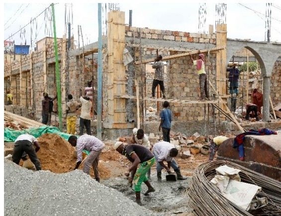
Construction in Baidoa (South West State): reinforced concrete as bearing structure and stone as infill for walls (CC - AMISOM)
