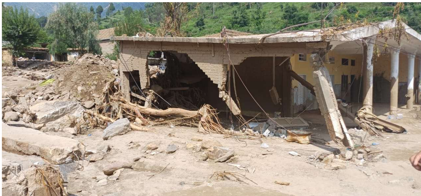
A house collapsed in Beshoni village, Buner district, KP (Credit: Umer Dil, District Coordinator, Buner)
