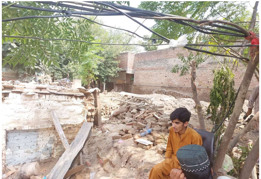
Village Council Mullababa, Tehsil Babozai, Swat district: Home to approximately 200 families received significant damage during the recent flash floods. The area was submerged under 8 -10 feet of water, resulting in damages to houses, schools; leaving areas filled with mud and debris. With the support of the government, volunteers, humanitarian partners (NGOS), residents are actively engaged in cleaning debris and repairing their houses and community infrastructure (Photo Credit: Saminullah Afridi, District Coordinator, Swat)
