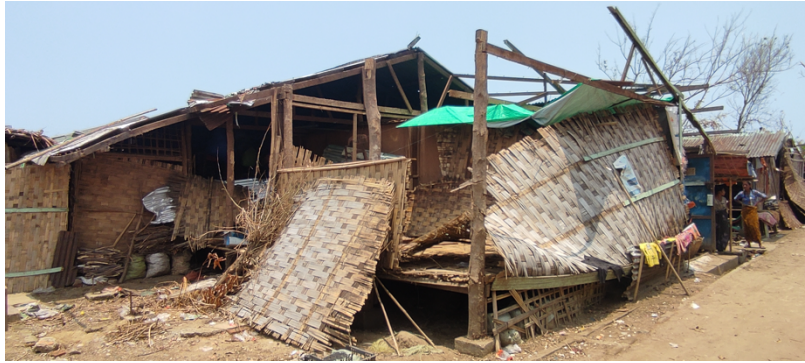
Photo 1: A severely damaged longhouse shelter in Dar Paing Rohingya camp in Sittwe Township.
