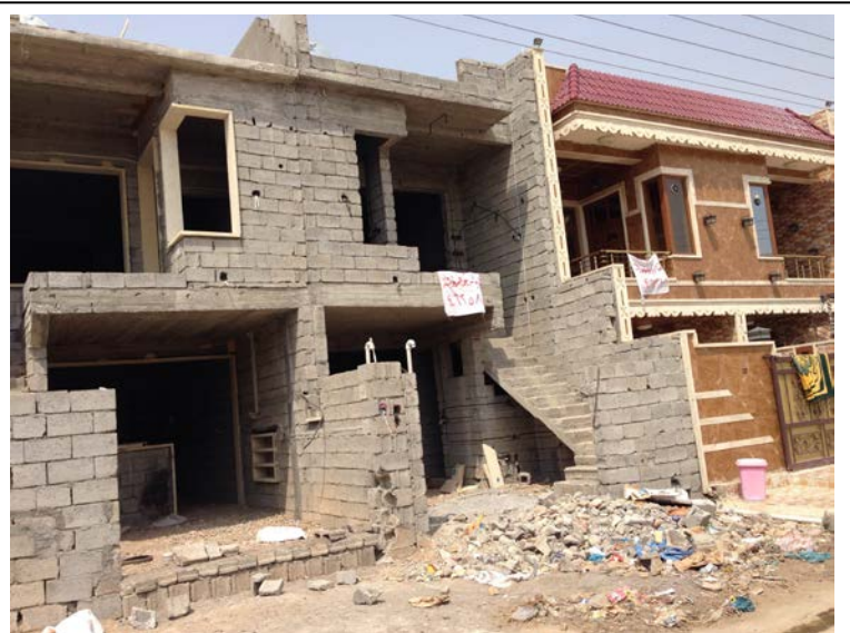
Example of a house in Beneslawa. On the right is a completed house, and on the left are two in need of upgrades.
