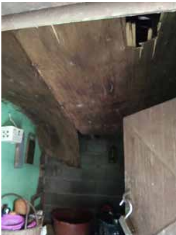
A roof collapsing in Bafoussam 3.
