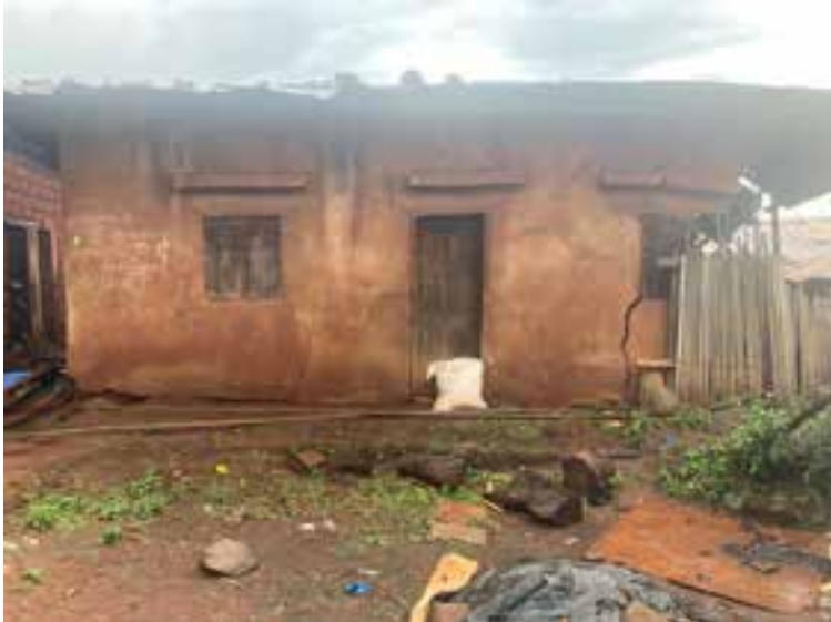
Shelter observed which had foundational risks where a family with many protection issues was residing.
