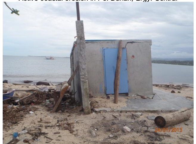
Effects of liquefaction in Block 7, Brgy/ Lambajon
