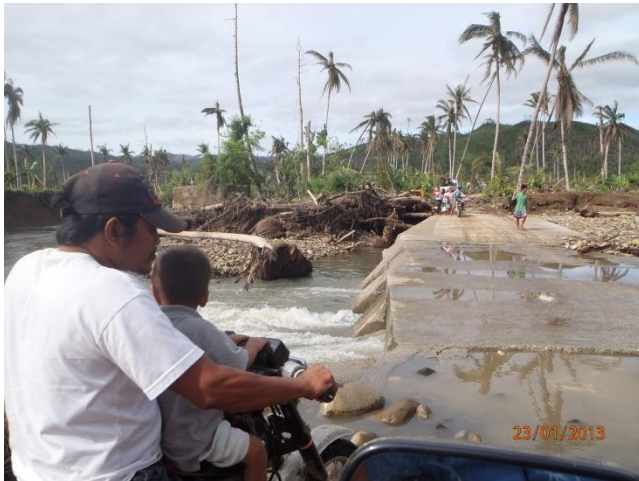
Spill way of Olin Creek, in So. Olin, Brgy. Mahan-ob. Water regularly overflow in this area during heavy precipitation or long duration of rain
