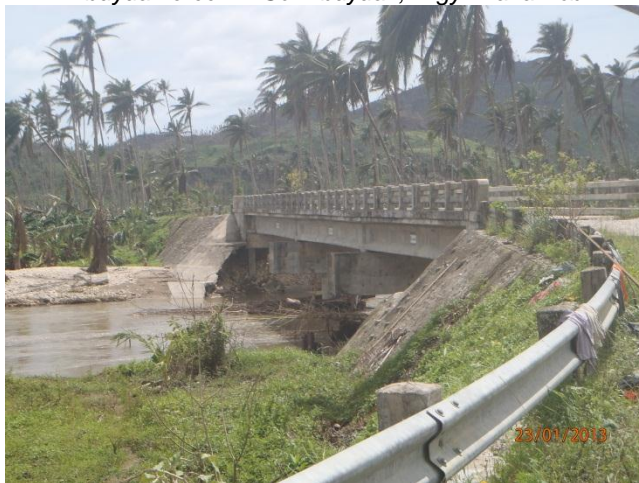
Scoured footing at the aproach of the bridge to Brgy. Batiano
