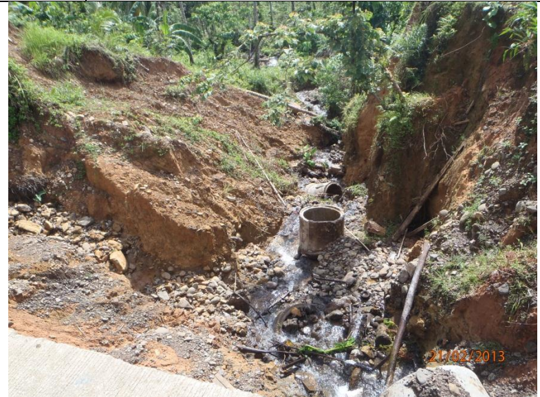
Earthflow and gully development in Po. Baclinan 2 along the national highway (Looking southeast; GPS location: 7°53'29.765"N 126°21'6.383"E)
