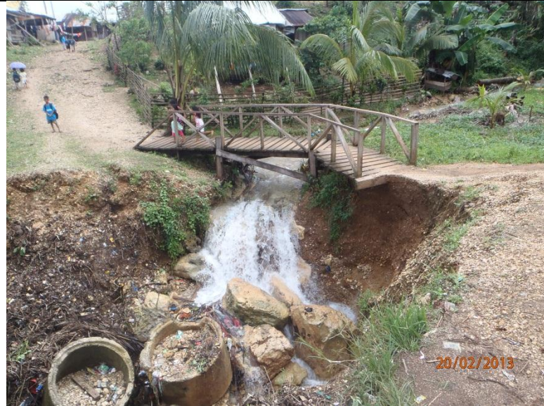
Washed-out culverts along Tugop Creek. Active scouring noted (Looking east; GPS Location: 7°52'55.387"N 126°14'58.213"E)
