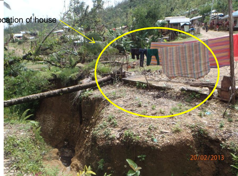
Scouring along the bank of a perennial creek in Po. 3 where 1 house was washed away during Typhoon Pablo. (Looking east; GPS location: 7°52'55.404"N 126°14'57.253"E)
