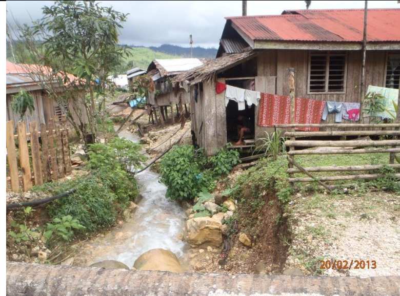
Houses in Po. 2 proximal to Tugop creek which are regularly flooded (0.5 m flood height) are subject for relocation (Looking north; GPS Location: 7°52'53.365"N 126°15'0.32"E)
