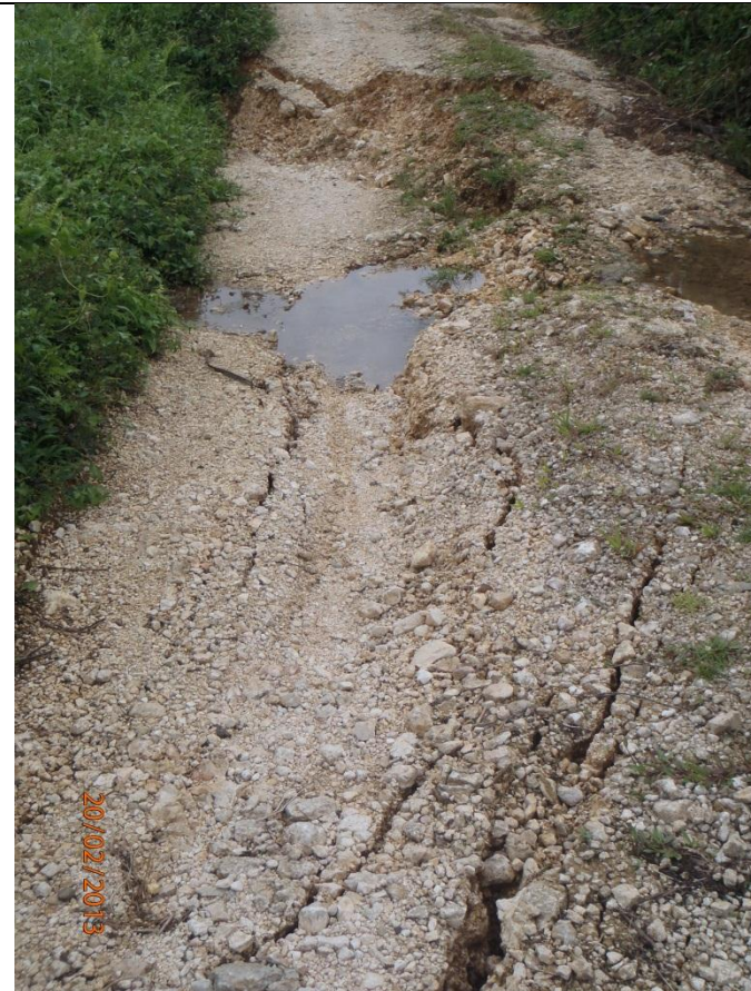
Tension cracks noted along the road going to So. 5M, Vertical displacement of 10 cm and horizontal displacement of 5 cm. Surface water is noted to seep into the cracks (Looking southwest; GPS location: 7°54'37.438"N 126°18'33.114"E)
