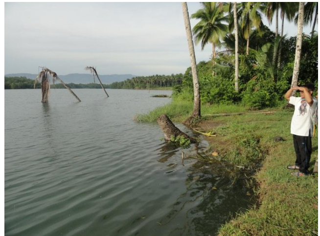
Scoured river bank and water level of Cateel river during high tide in So. Panan-awan
