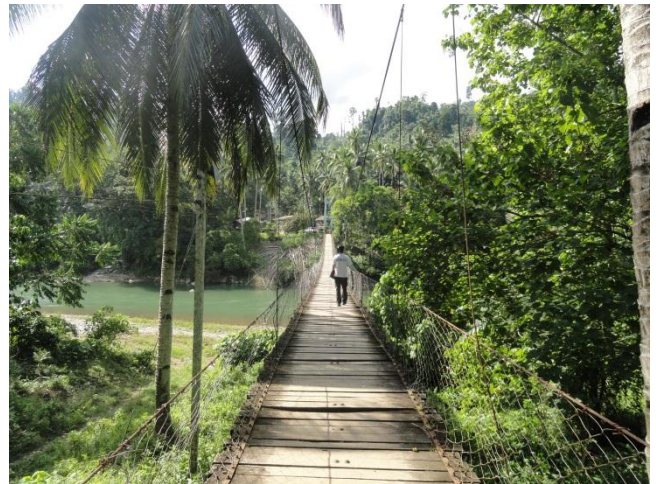
Previously damaged hanging bridge by floodwater in Brgy. Maglahus
