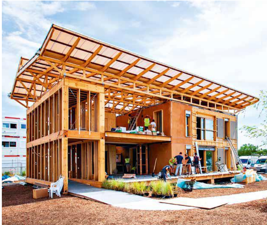
Terra Nostra, prototype of economic housing. Prefabricated in 4 months by students of ENSAG in 2016
