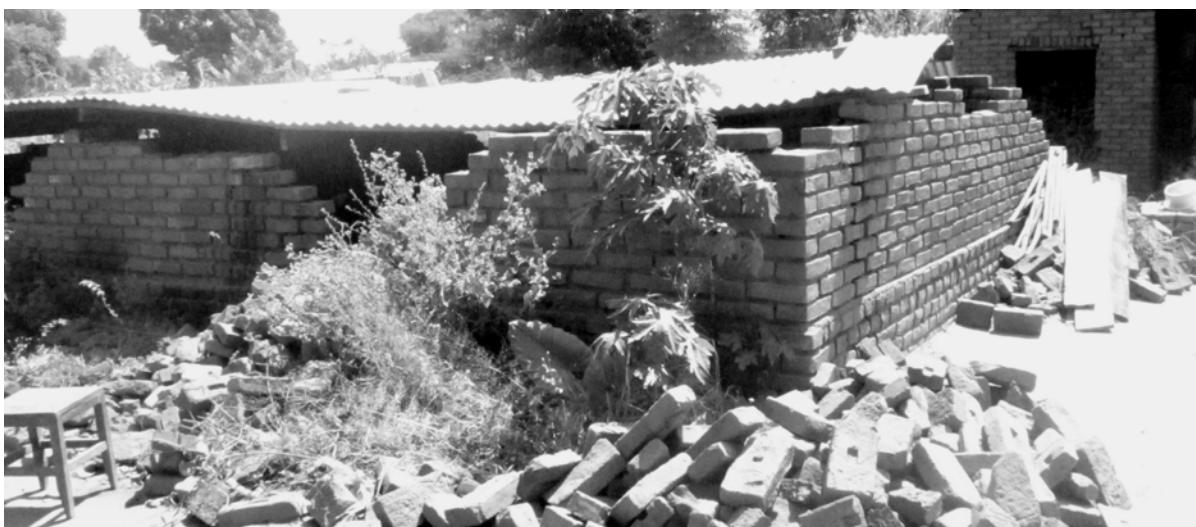
Fig1. One of the damaged houses in the 2009 earthquake, Karonga District
