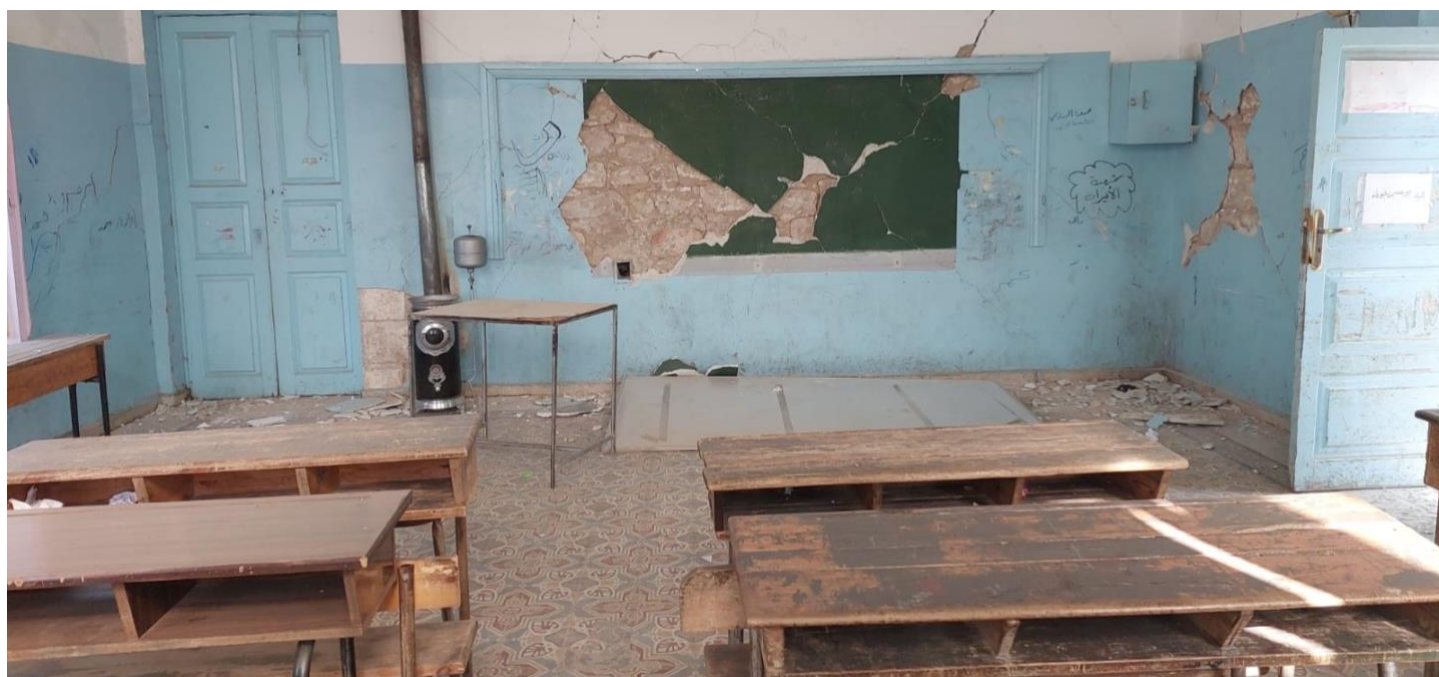
Some schools in Harim in Idlib are over 100 years old, making them highly vulnerable to earthquakes. Students from this damaged school were luckily transferred to another school. 27 February 2023. Photo credit: HFOs
