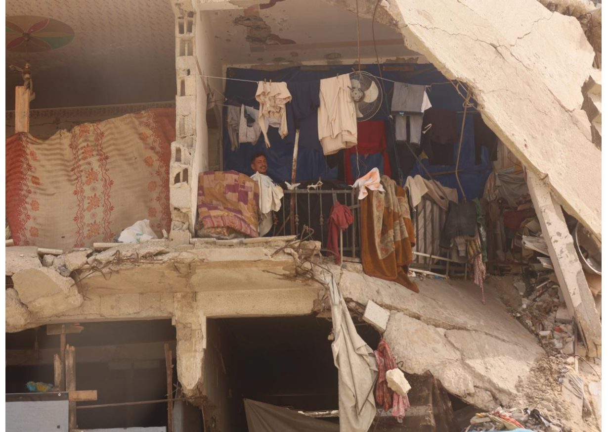
Damaged housing unit - Source: IOM.
