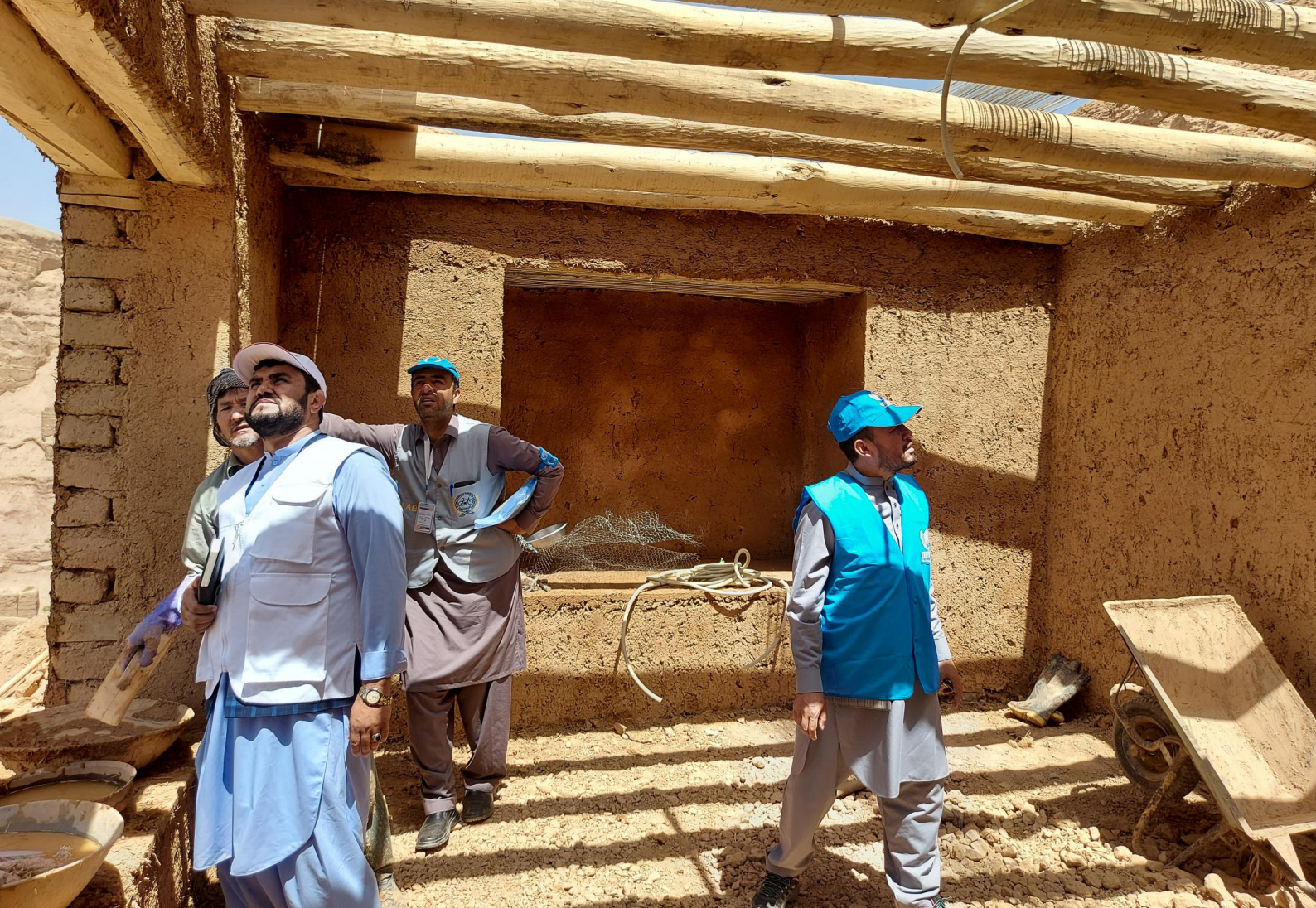
Monitoring of Transitional Shelter in Bamyan province . Photo taken by shelter Cluster , October 2022
