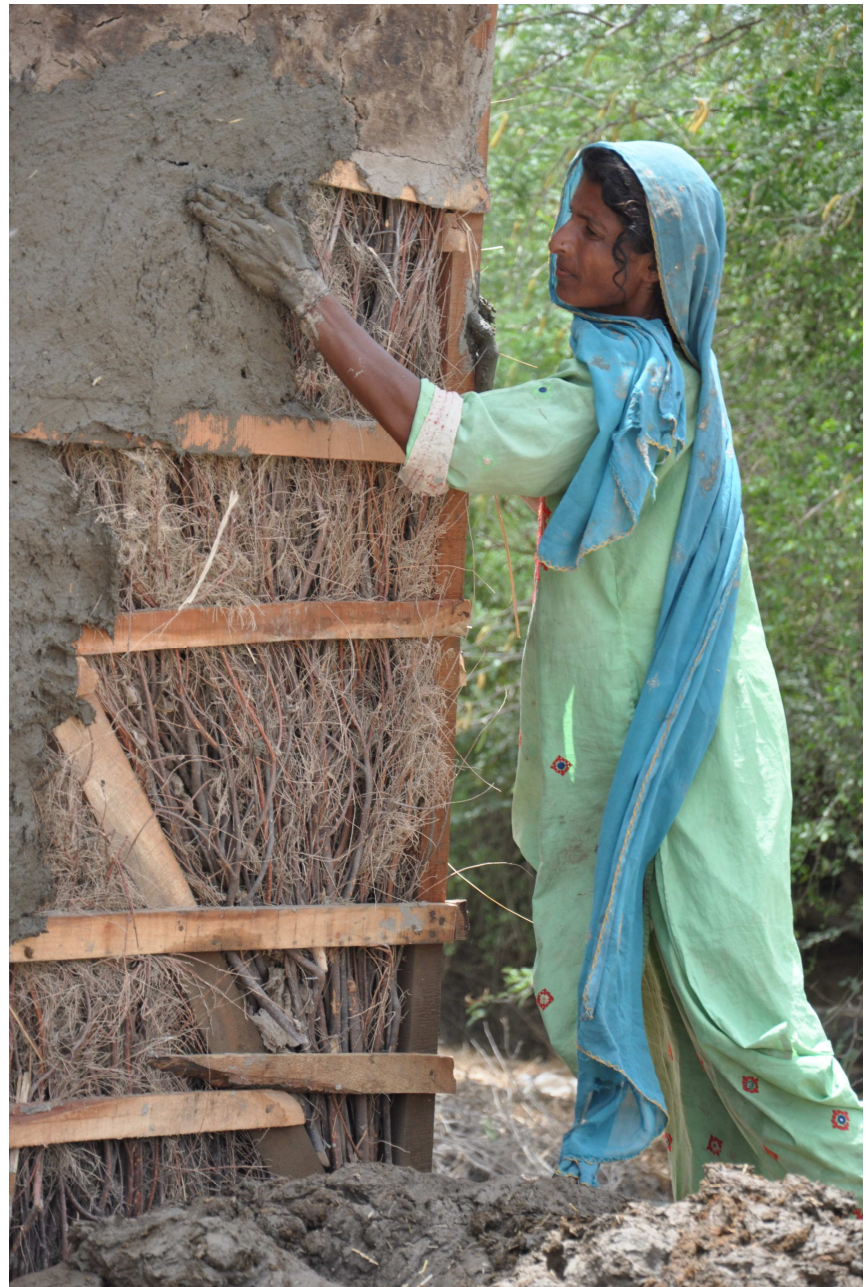
A woman helps construct her home following the 2010 Pakistan floods. Photo: IFRC/Rabia Ajaib
