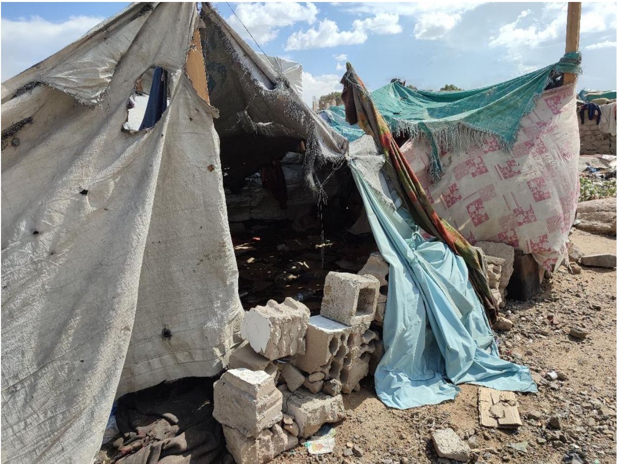
An emergency shelter severely damaged by ongoing floods in Sa'adah District, Sa'adah Government . © YDF/ Mohammed Haikel
