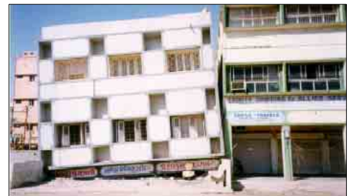
Fig 4.17: Collapsed soft stories
