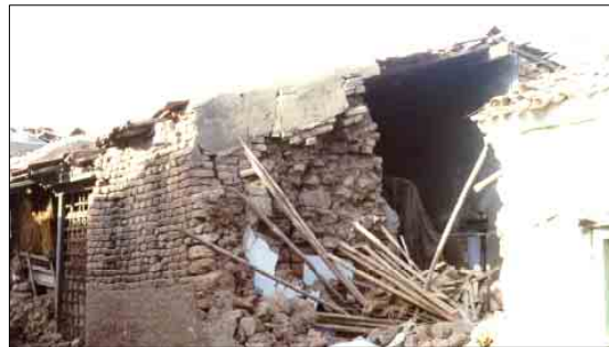
Fig 4.7: Collapsed Unreinforced brick house
