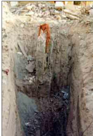
Fig 4.13: Absence of plinth beams
