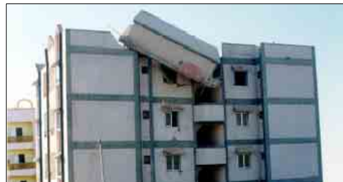
Fig 4.16: No Support for rooftop water tanks
