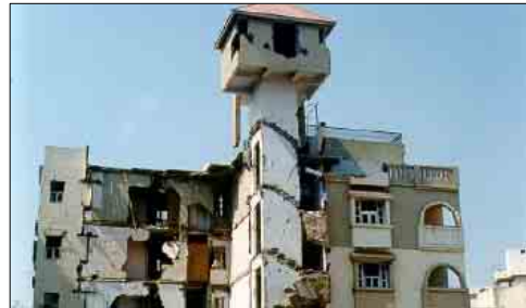
Fig 4.15: Inadequate transfer mechanism
