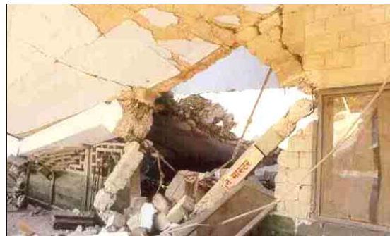
Fig 4.8: Collapsed Cement Block masonry structure
