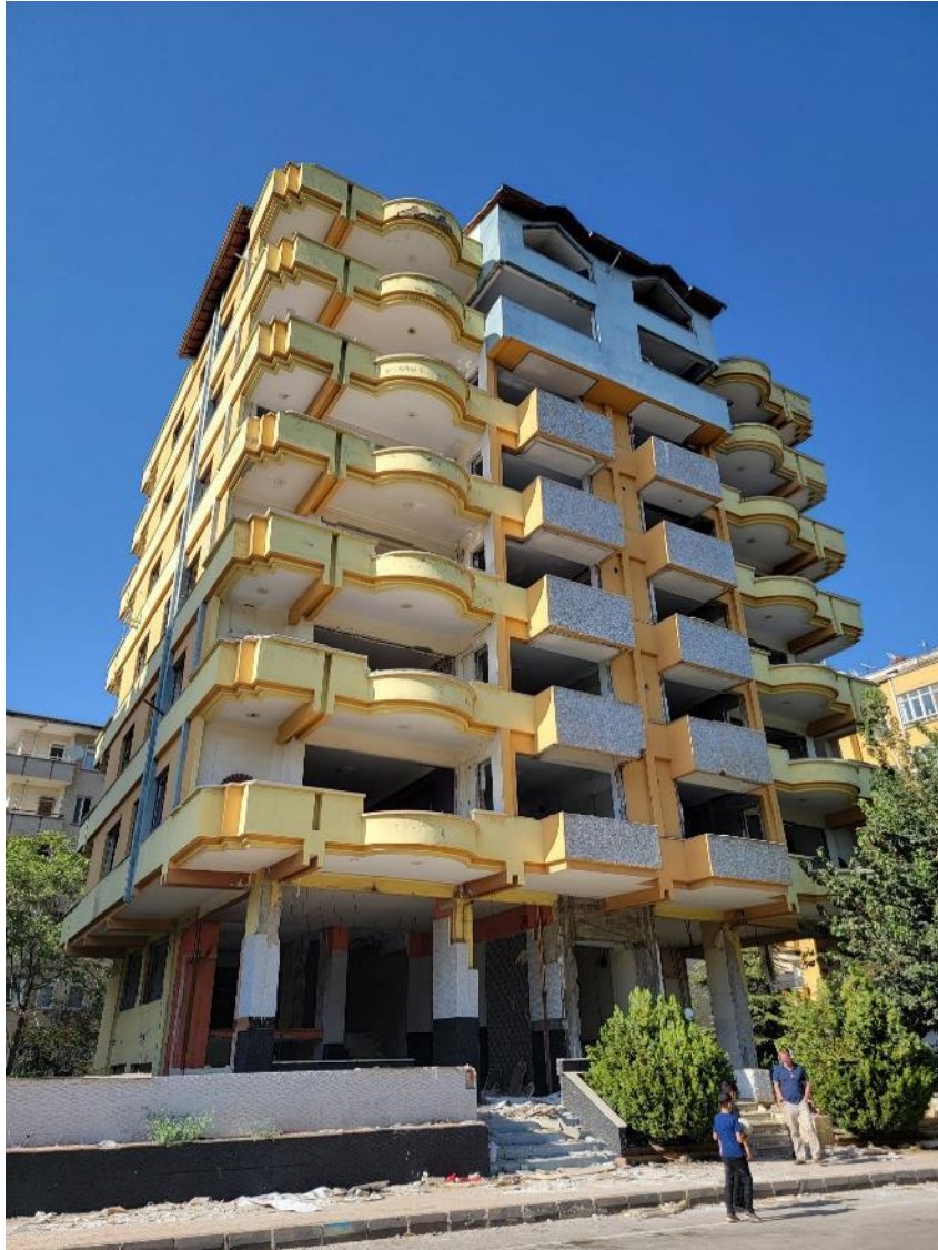
Building with medium damage
