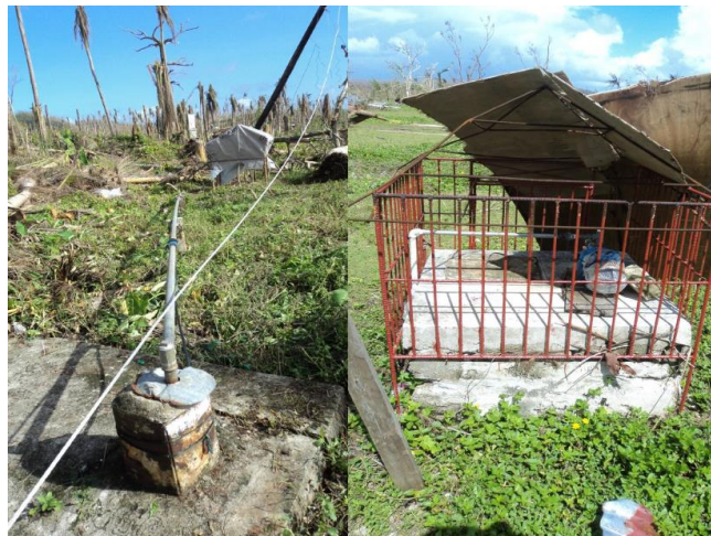
Figure 12: Level II WSS not working due to interrupted power supply
